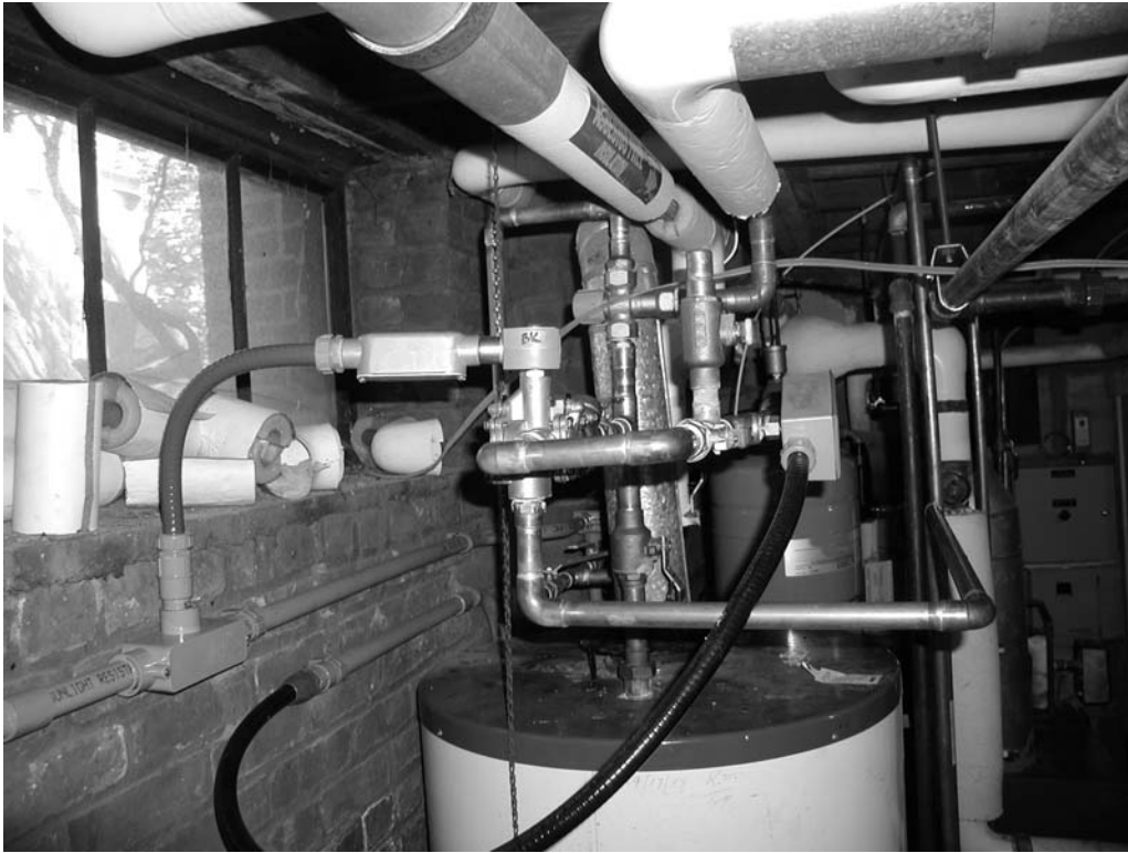
Figure 3. Complex piping required near domestic hot water tank in residence 3.
