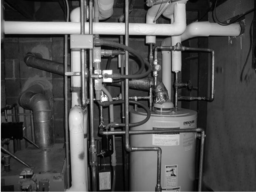
Figure 1. Complex piping required near domestic hot water tank in residence 1.
