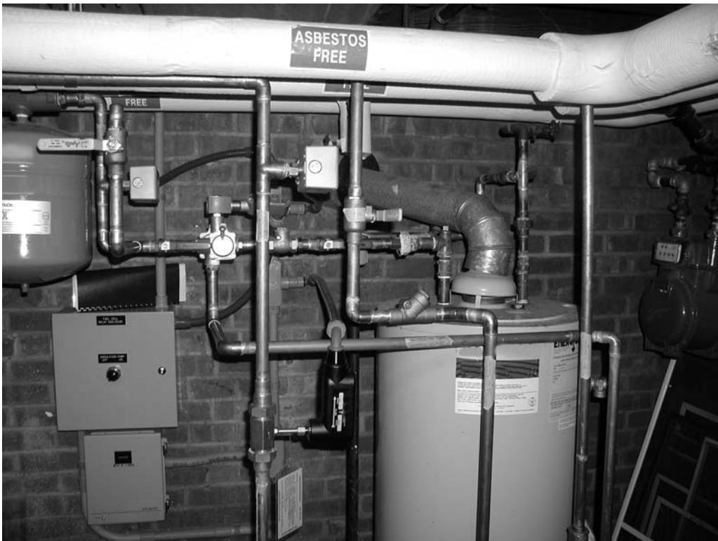
Figure 2. Complex piping required near domestic hot water tank in residence 2.
